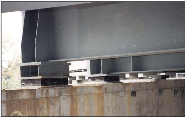
Building Support Steel on 6.5 Hz Rubber Bearing Pads
