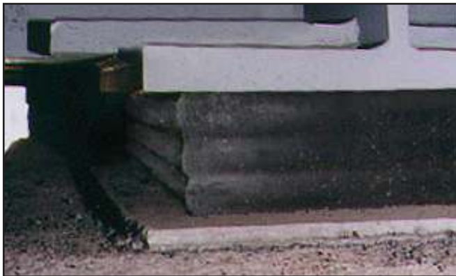
Loaded Bearing Showing Bulges Between Plates
