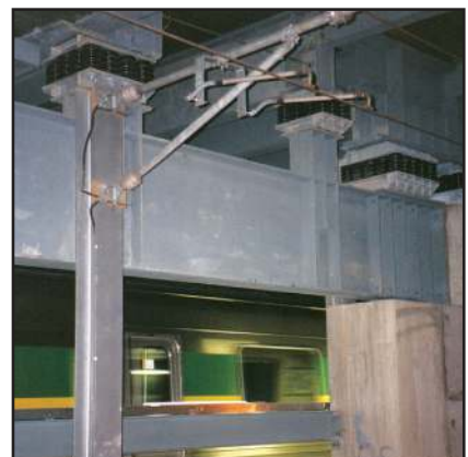
Train Passing Immediately Adjacent to Building Columns-Note Spring Isolation on Top of Column
